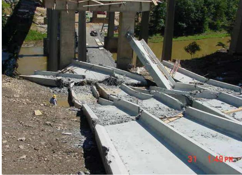
Figure 1.2 - Collapse of I-80 girders in Pennsylvania (Hurff, 2010)
